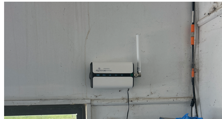
Mulesight Gateway installation
